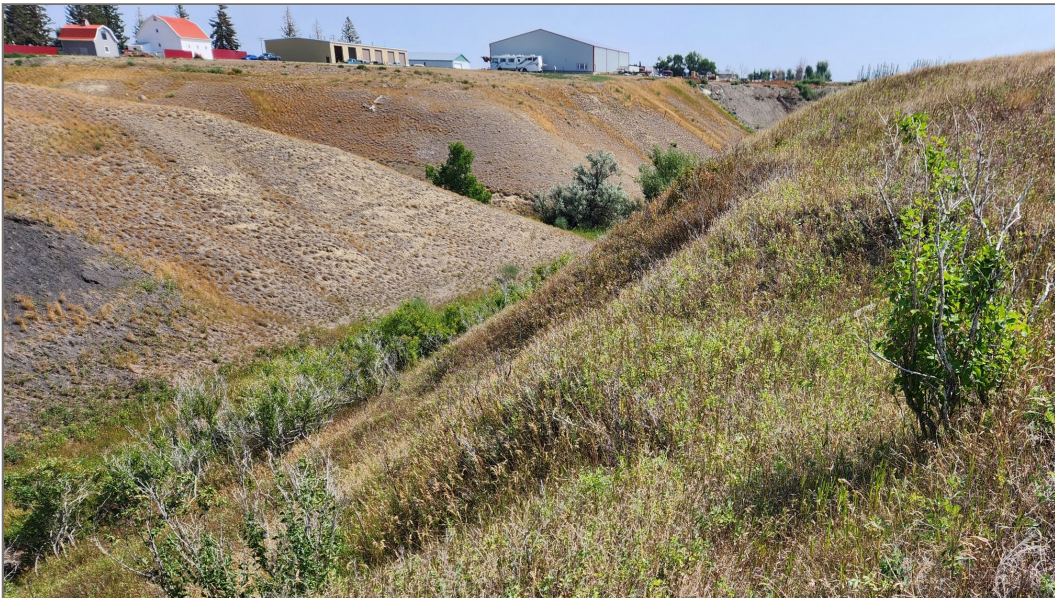
Photo 8: Historical Instability on Slope North of Site – Facing East.
